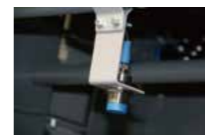
Step missing detect
